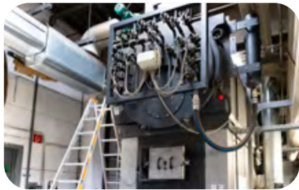
Wood-burning heating system
