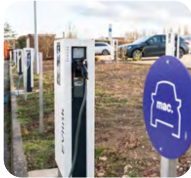
EV charging stations
